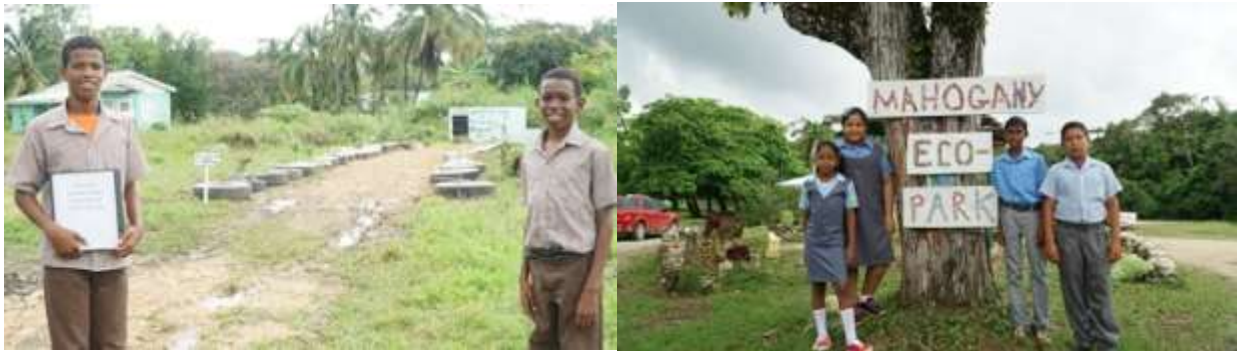
Picture above: Renovation of concrete garbage bin and establishment of an eco-park for outdoors learning.
