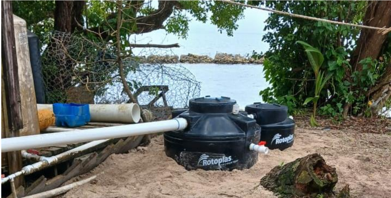
Figure 15: Showing the new wastewater treatment system
